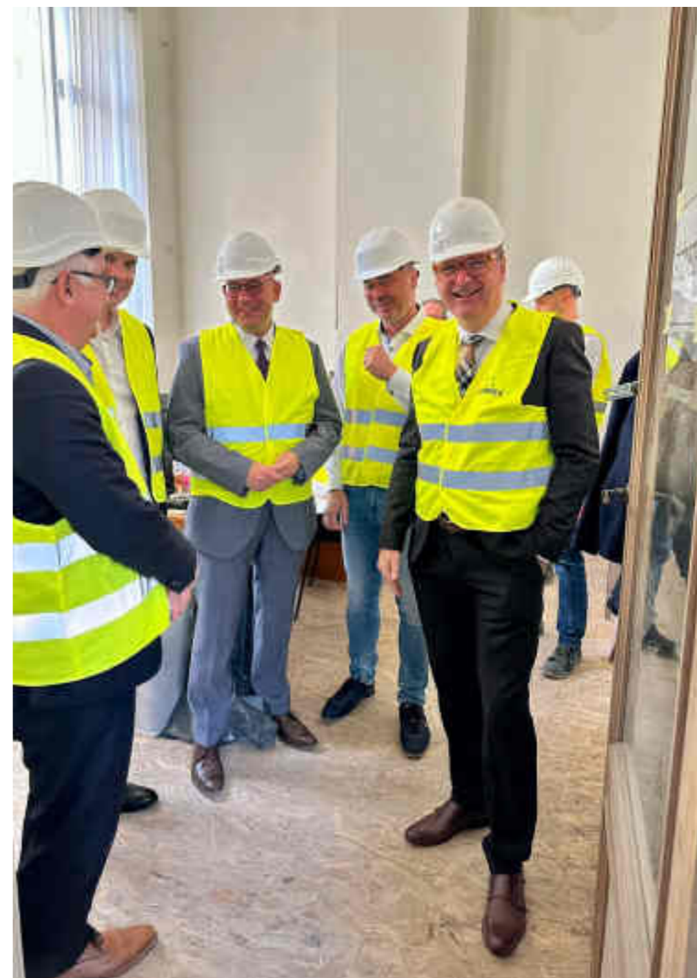
The House of Hungary conveys the values of Hungary's rich culture. Csaba Káel (on the right) is seen here during the construction.
